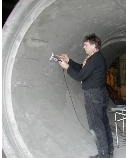
Delaminations in sour pipes, Denmark
