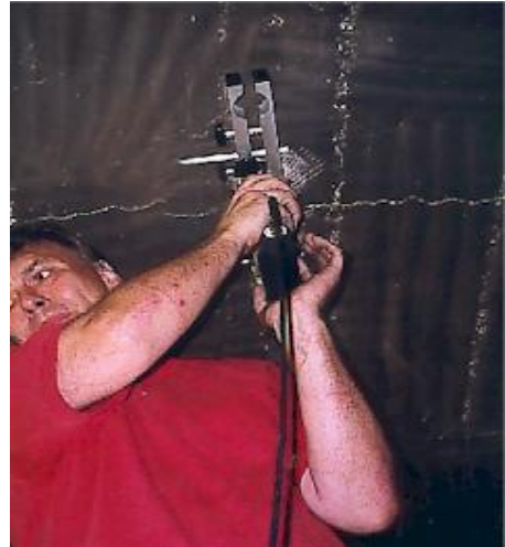
Depth of surface opening cracks in a fire damaged slab, Germany
