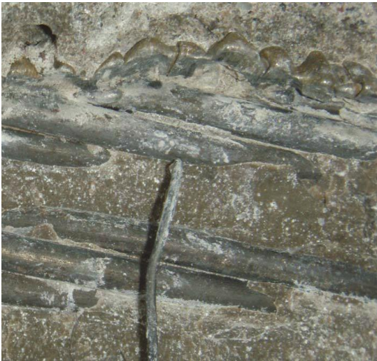
Fig.3 Sound strands in well injected duct
