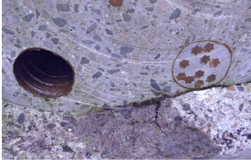
Figure 21. End cut in the slab for illustration of the empty duct and the injected duct with the 10 strands
