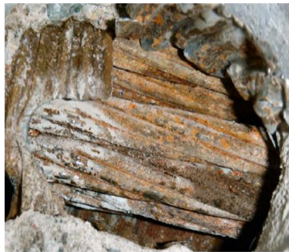
Fig.4 Corroded strands in empty steel duct
