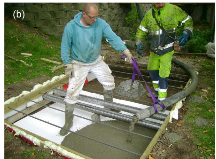
Figure 9. (a) Slab formwork with ducts and bars installed; (b) placing the self-consolidating concrete.
