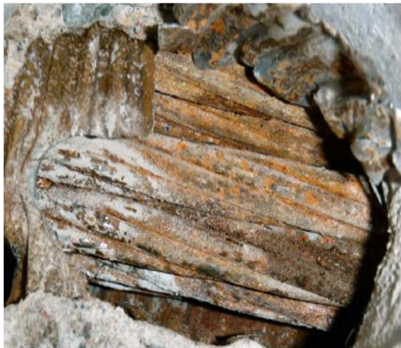
Figure 4. Corroded strands in an empty steel duct.
