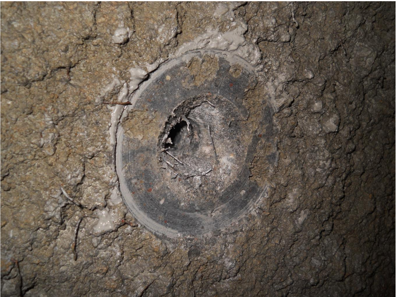
Capo-Test failure on shotcrete with steel fibers
