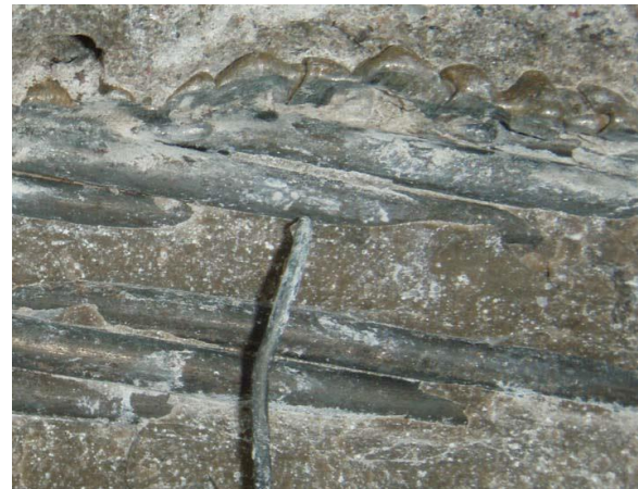
The excavated duct at location (1) reveals that some of the strands are not embedded in grout
