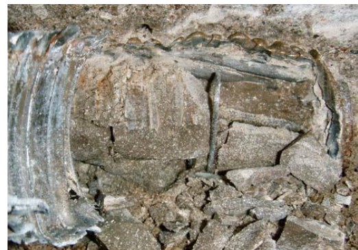
B-scan at location (2) with no voids indicated in grouted duct. The excavation reveals the strands encased with grout; some of it was fractured in the process and this exposed some wires.
