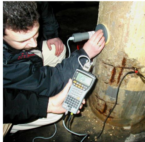
GalvaPulse (older model) testing in progress for corrosion activity of a heavily corroded column
