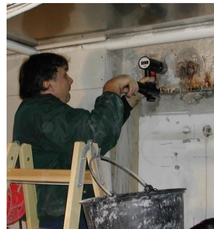
CAPO-TEST being performed in parking garage to evaluate in-place strength of suspect concrete
