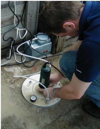
Routing recess for preparation for CAPO-TEST to evaluate surface strength of an industrial floor slab
